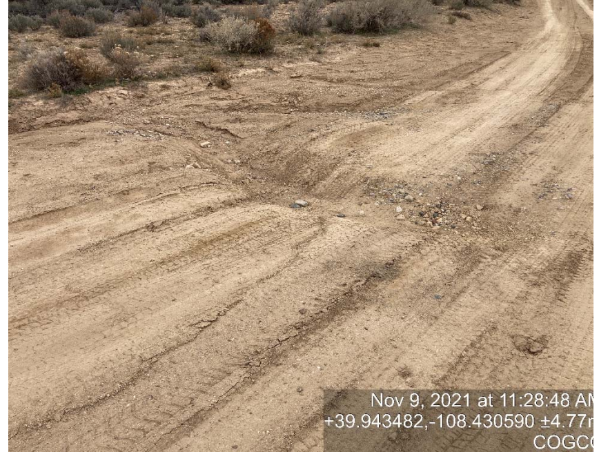
Lack of stabilization/erosion
