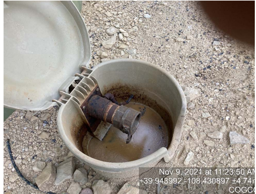
Load out lines missing caps/bull plugs
