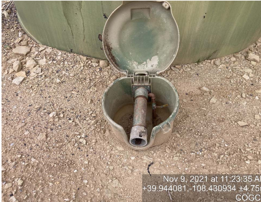
Load out lines missing caps/bull plugs
