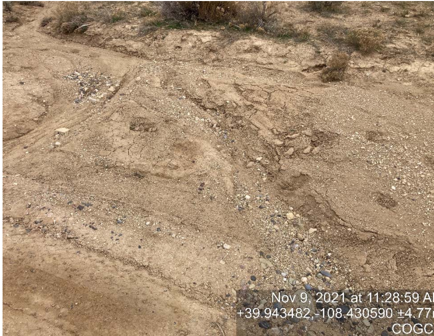
Lack of stabilization/erosion
