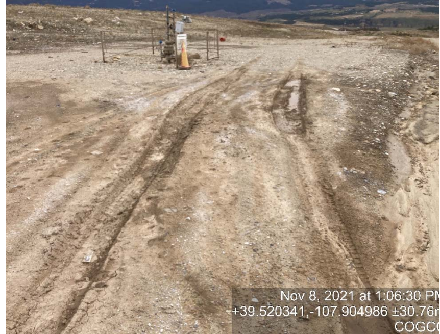
Lack of stabilization/compaction
