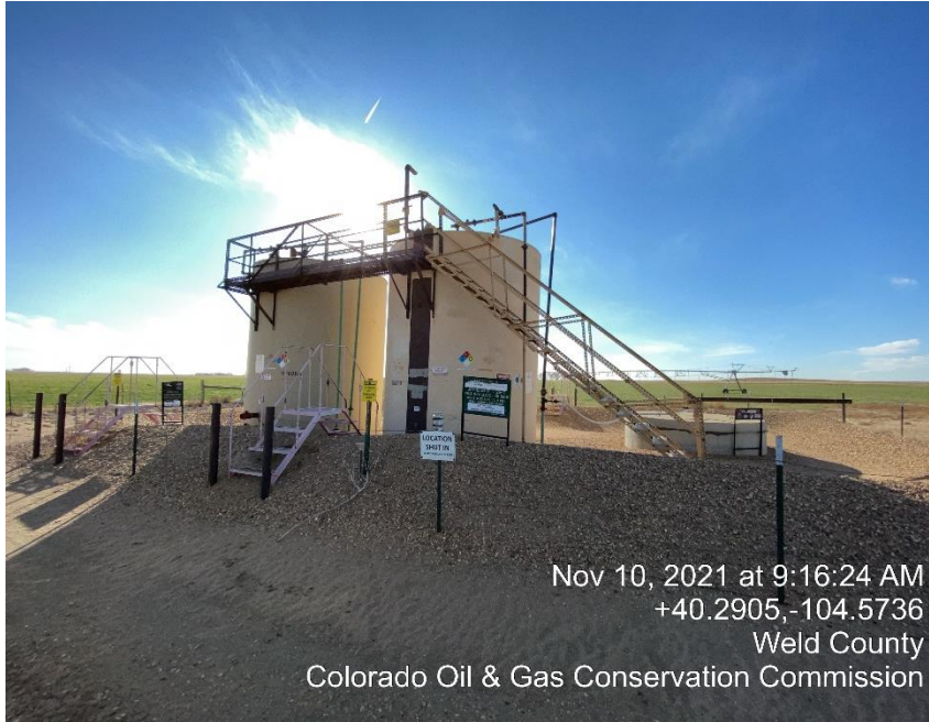
Photo #1 Tank Battery
