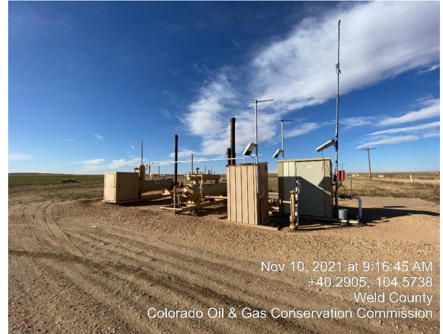
Photo #2 Production Equipment
