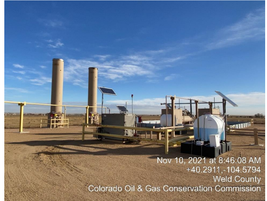
Photo #2 Production Equipment
