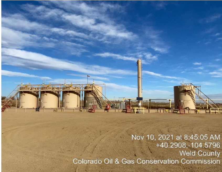
Photo #1 Tank Battery
