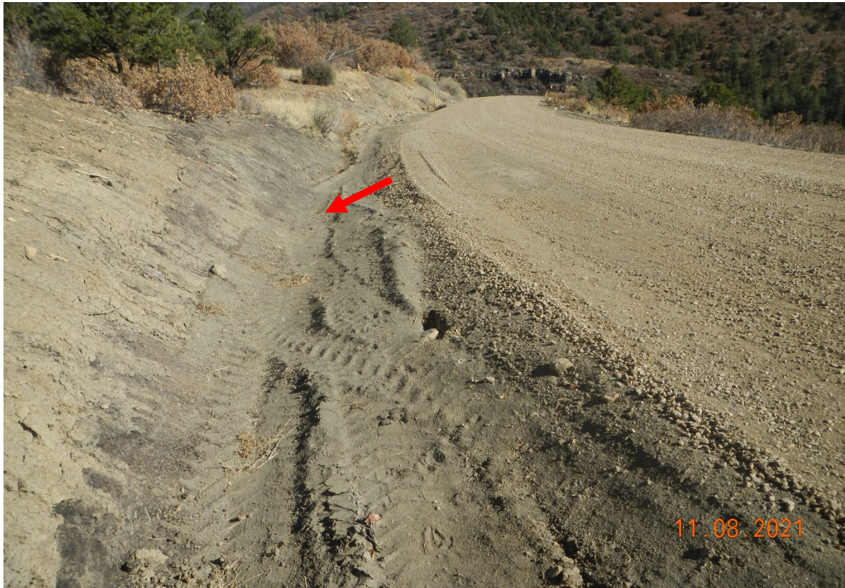
Photo 2. Facing back down the road. This steep area of the roadside needs additional BMPs' to prevent erosion and sediment accumulation at the culverts.
