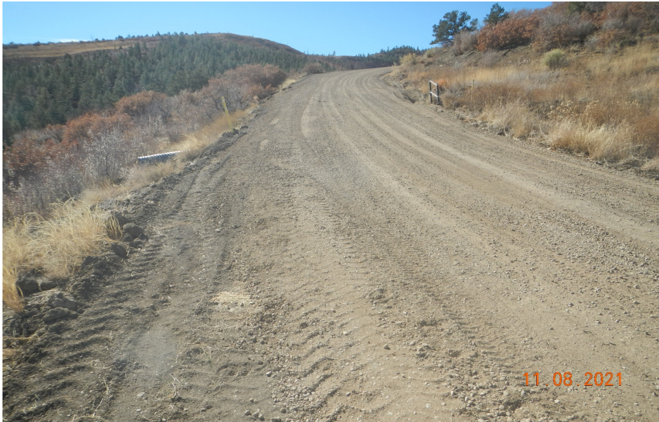
Photo 1. Facing southwest along the access road. The road was regraded and additional gravel was spread along the road.
