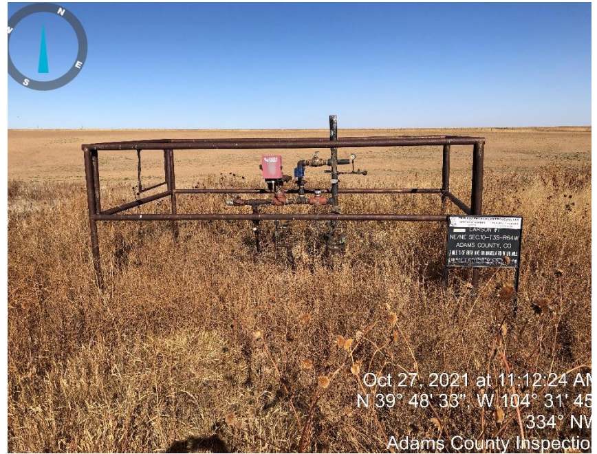
Photo #4 Well Head.
