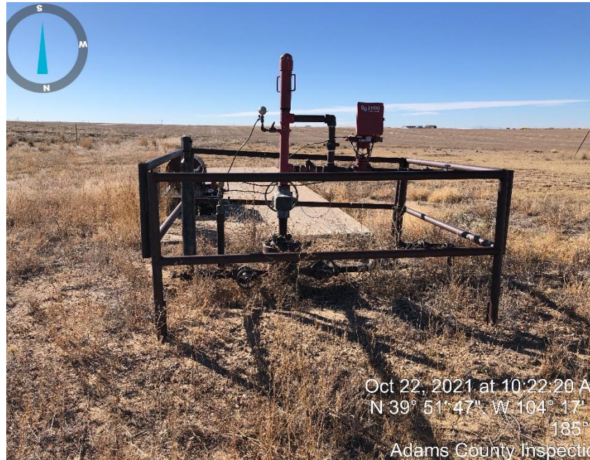
Photo #1 Well Head.
