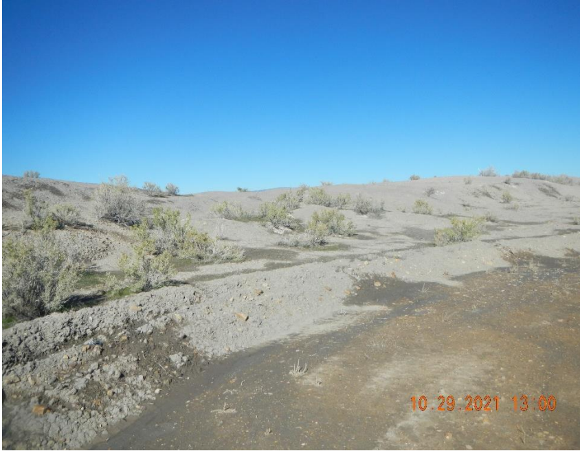
Sediment build up behind berm.
