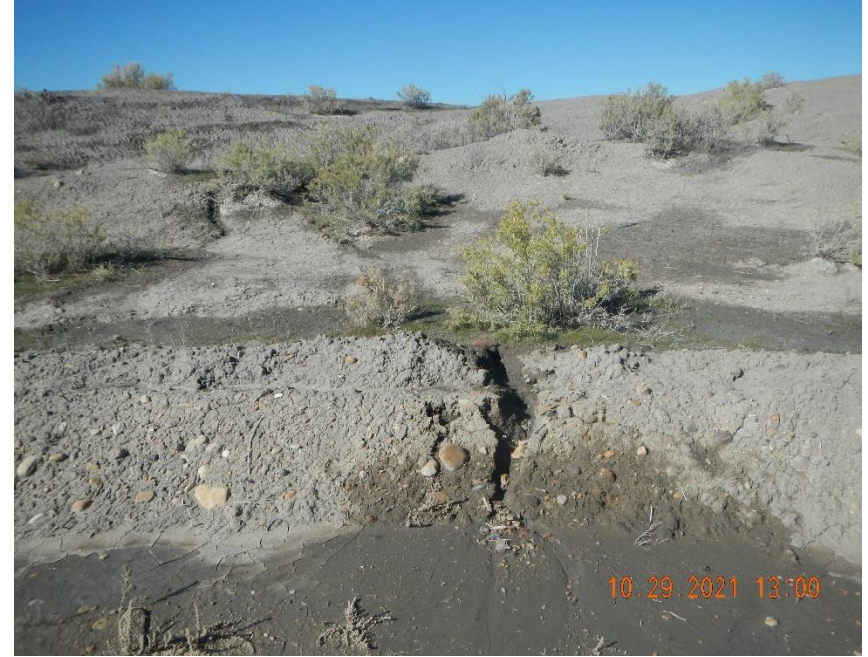
Erosion rill breaching berm wall.
