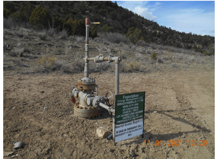
Wellhead with sign. Bradenhead plumbed to surface, CA completed.
