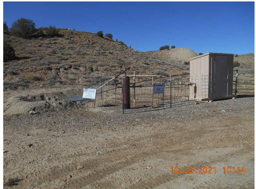
Meter housing with fence and sign.
