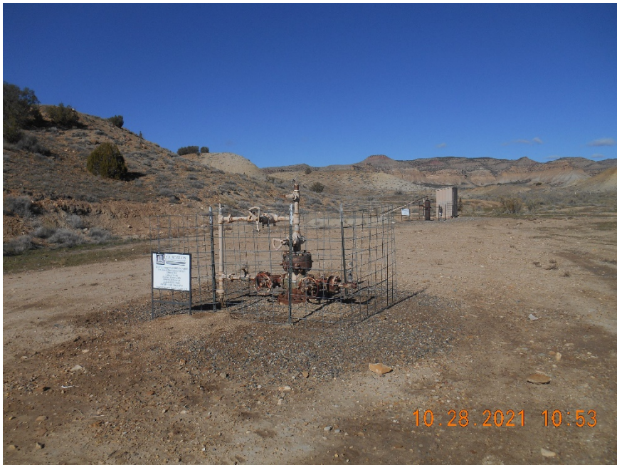
Wellhead with fencing
