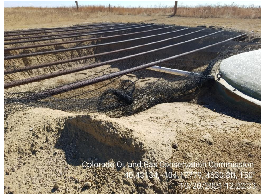
Photo 6 – Netting NOT secure
