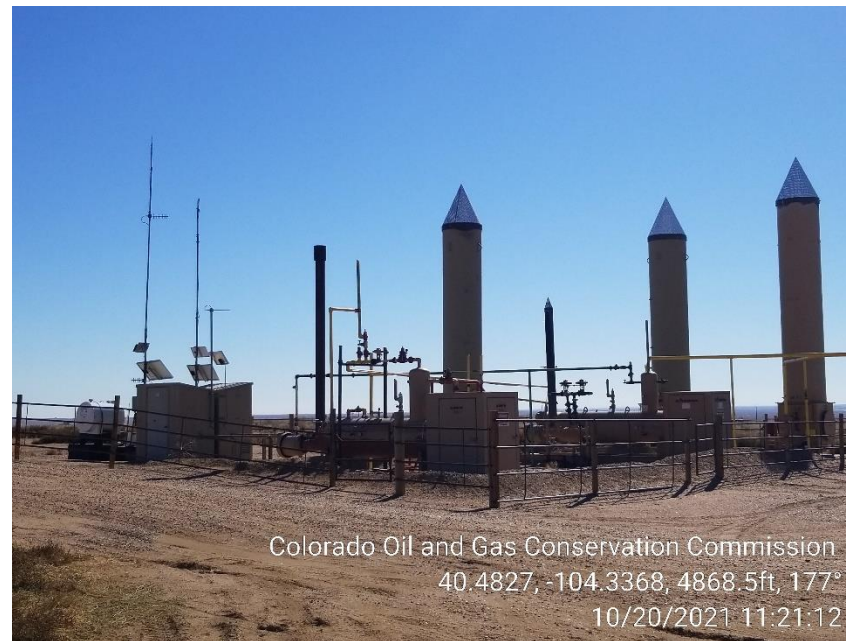
Photo 2 – Separators and ECDs
