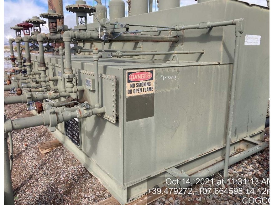
Lack of labeling
