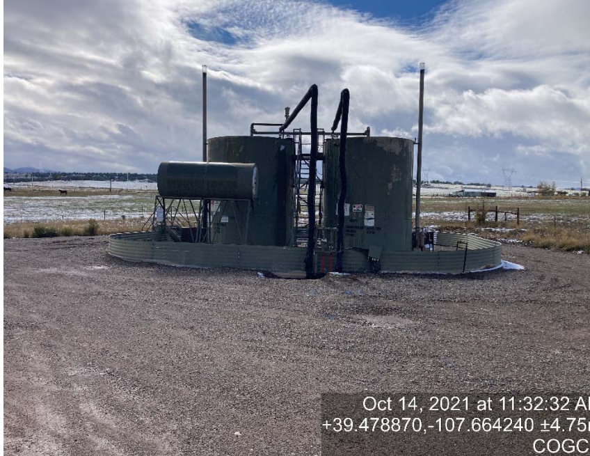
Location/lack of battery signage
