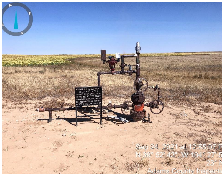
Photo #3 Well Head.
