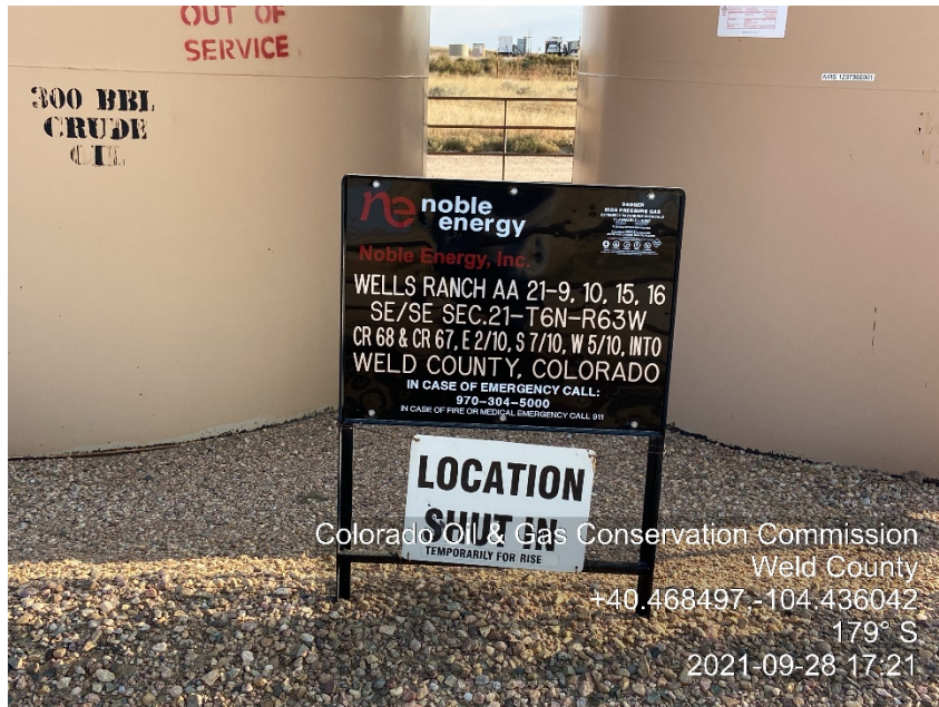
Photo #3 Wells Ranch AA 21-09, 21-10, 21-15, 21-16 Battery site Inactive | Shut-down Battery sign
