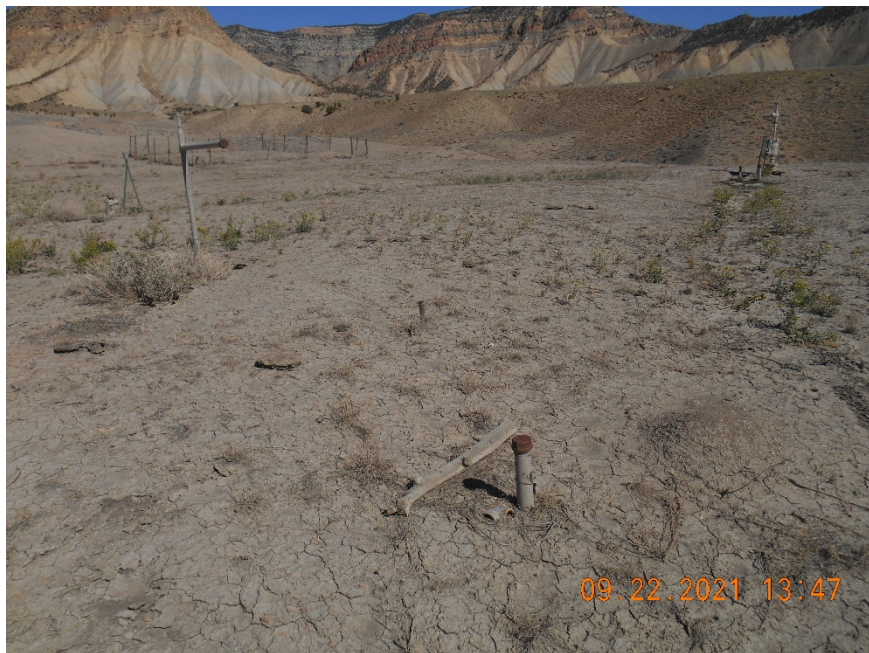
2- Disconnected 2" flowline. 1" flowline riser
