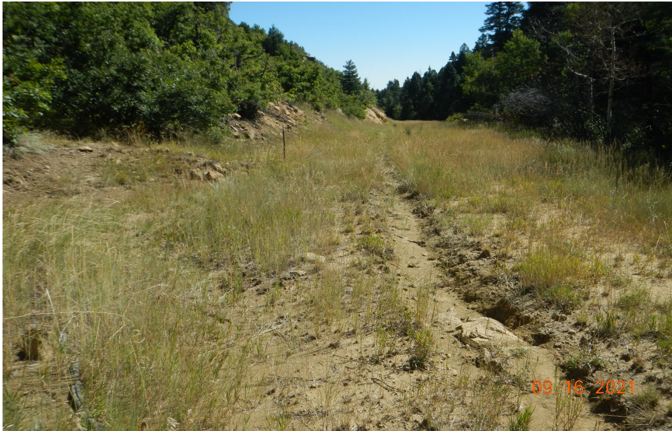
Photo 10. Facing east along the access road. It appears erosion has occurred along the road and stormwater is not diverted toward the culvert.
