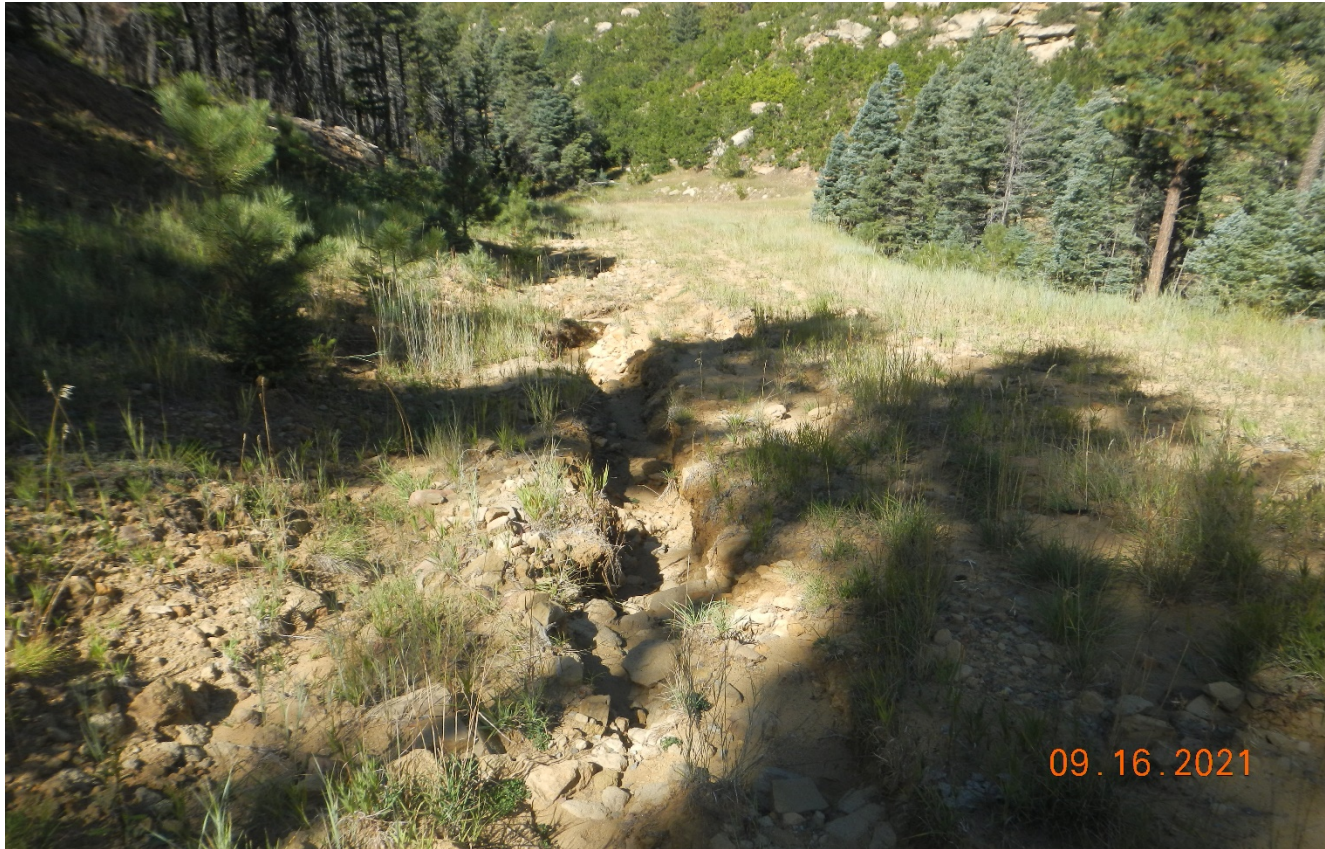
Photo 7. Facing northwest along the access road descending into the canyon. There is erosion along the road all the way down to the canyon bottom.
