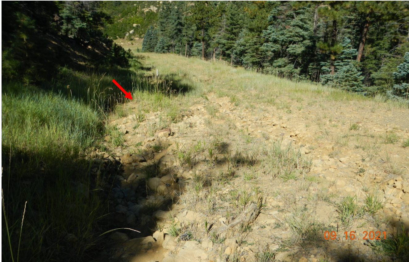
Photo 6. The arrow points to a culvert which is filled in with sediment.
