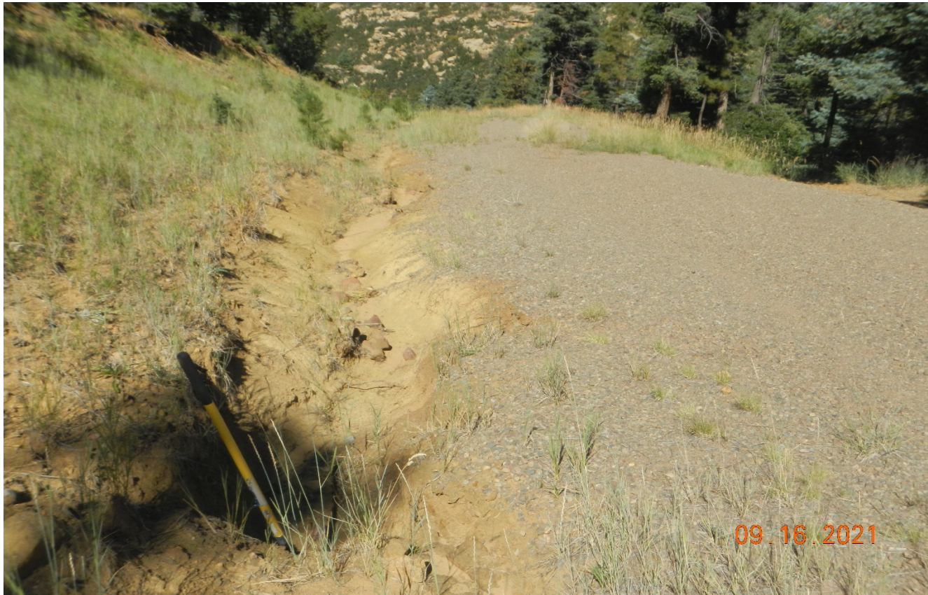
Photo 5. There is erosion occurring along the side of the road and culverts are filled in with sediment.
