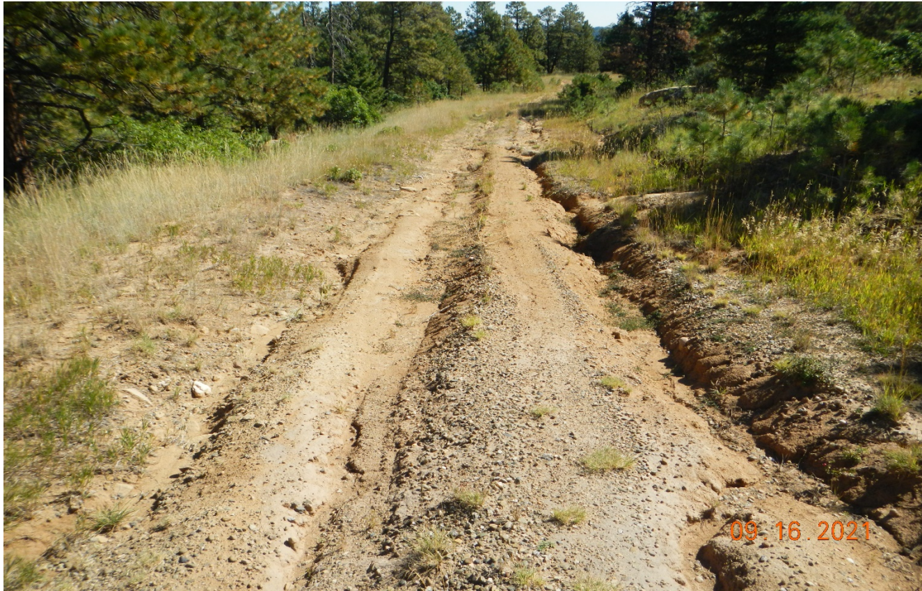
Photo 1. Facing northeast along the access road. The road is not stabilized and there is erosion channels along the road. Previous corrective action was not completed.
