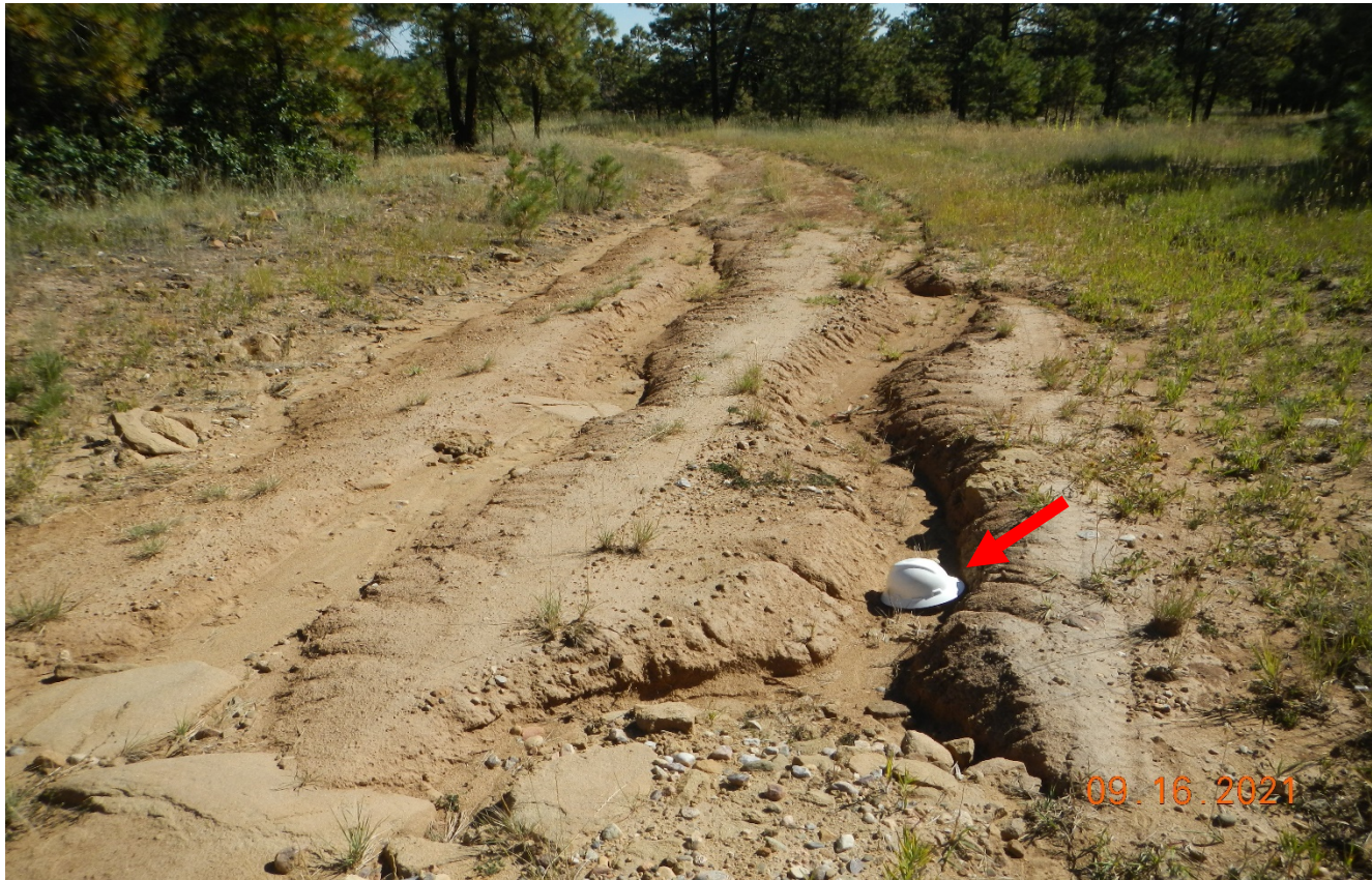
Photo 2. The road is not stabilized and there is erosion channels along the road. Red arrow points to hard hat for scale. Previous corrective action was not completed.
