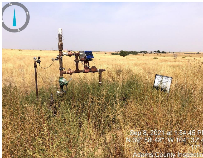
Photo #1 well Head.
