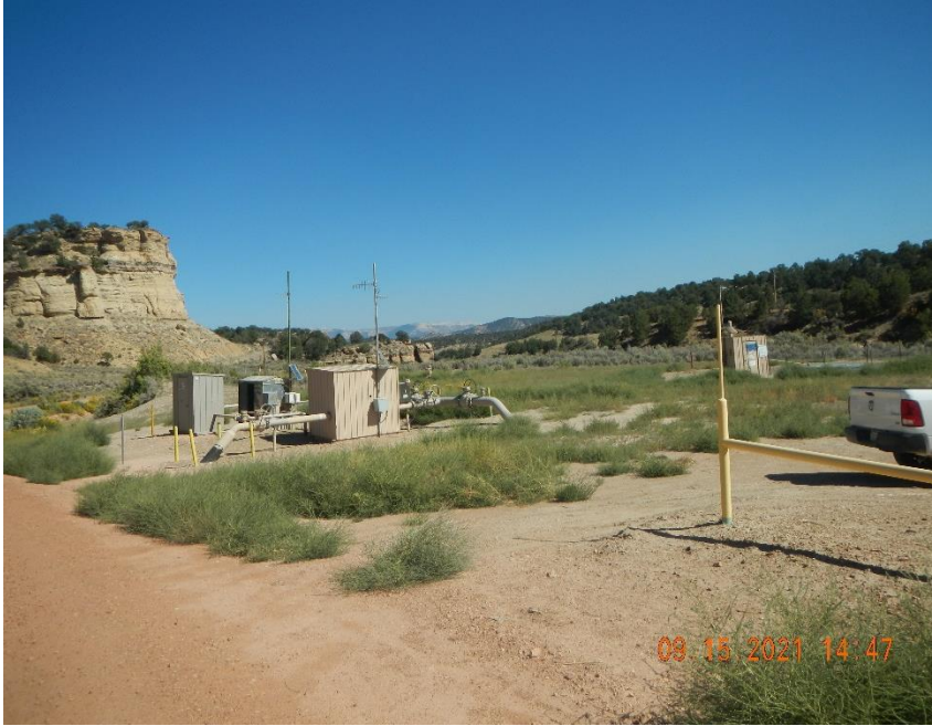
Dead weed debris covering location.
