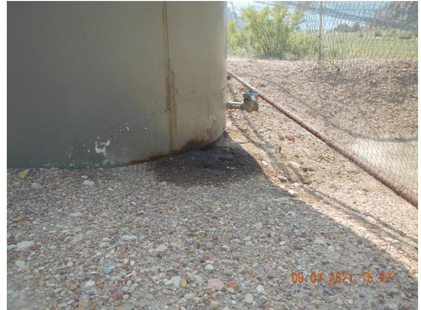
Spill hydrocarbon fluid on tank berm floor.
