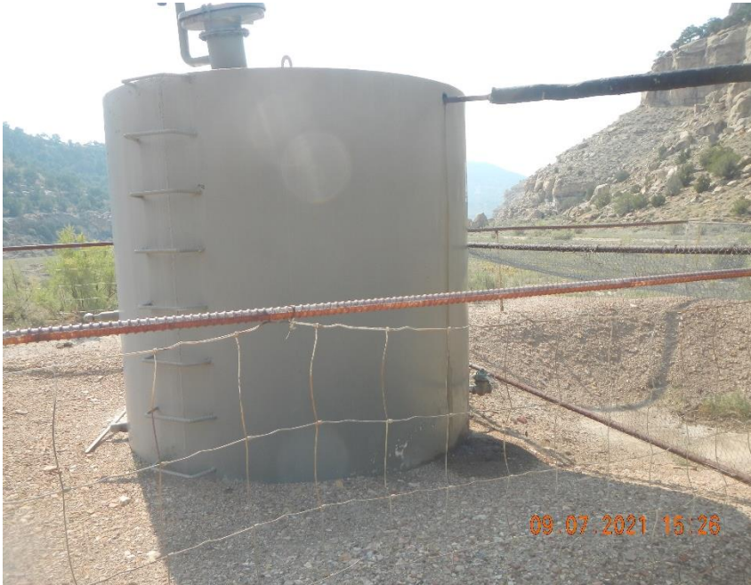
Tank fluid contents leaking from open hole that flow line is running into.
