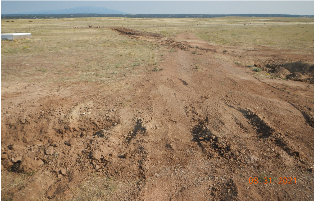
Photo 1. Facing north along the access road. There was recent disturbance from what appears to be a surface owner water line.
