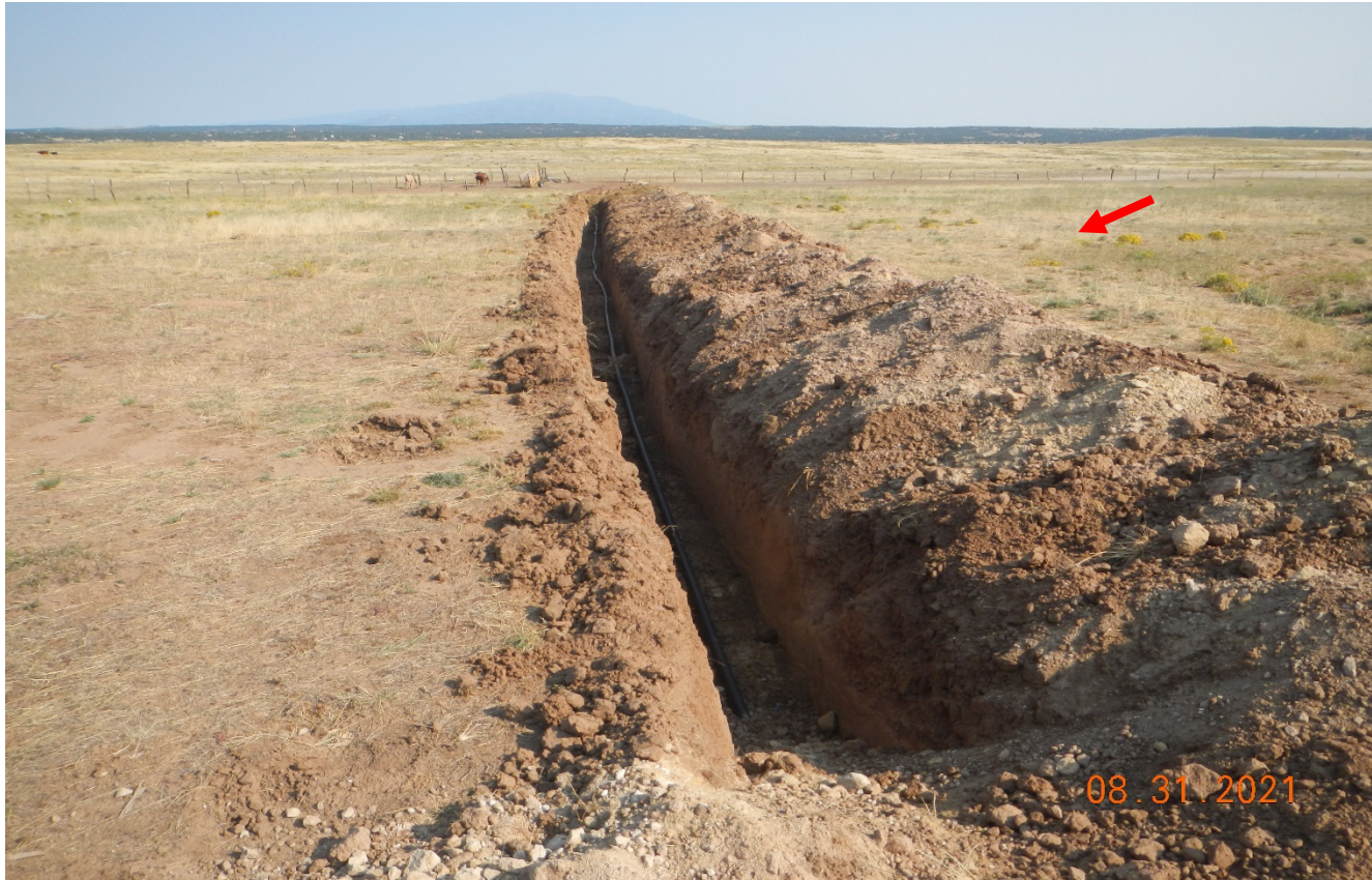
Photo 2. A trench was dug through the center of the location. Red arrow points to area of the abandoned well.
