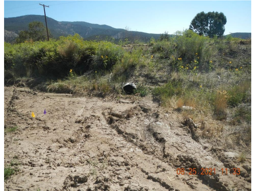
Released fluids travelled beneath Highway 151.
