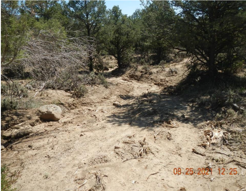
Impacted material in natural drainage.
