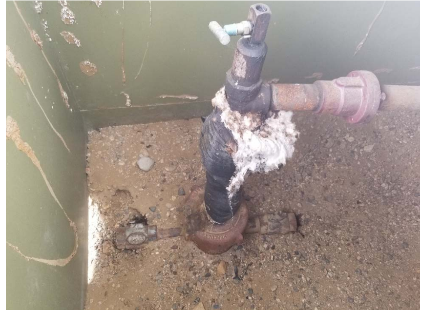
Photo 2. No bradenhead access apparent.
