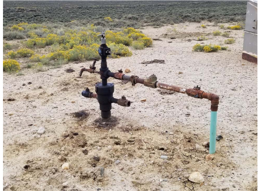
Photo 2. No bradenhead access apparent. Stained soil at wellhead.
