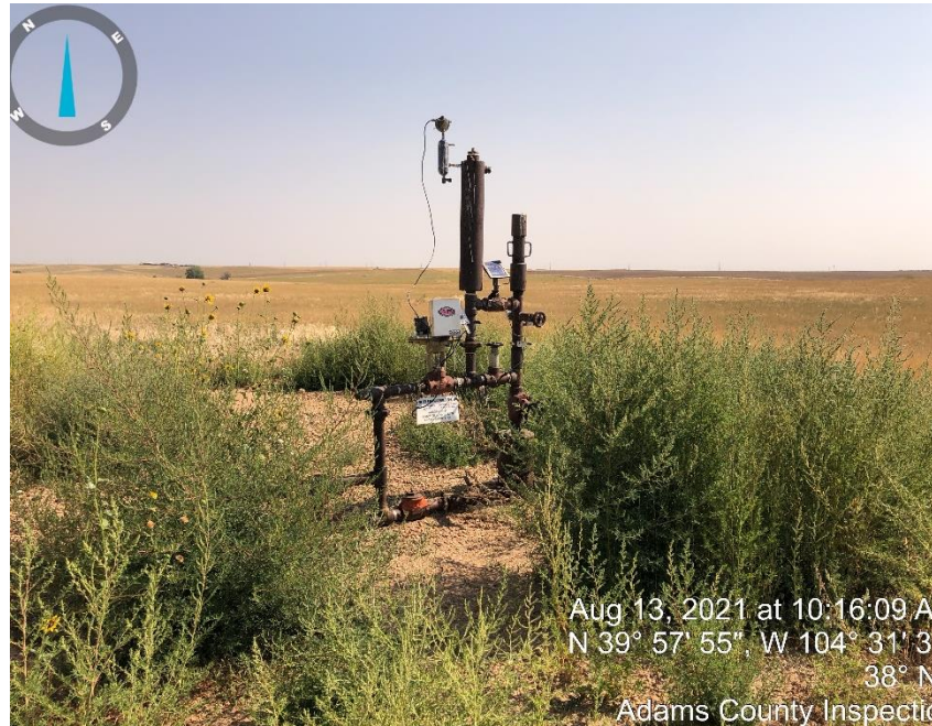
Photo #3 Well Head.
