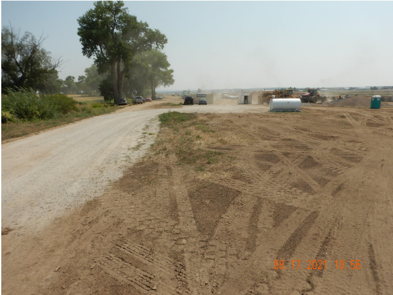
Photo 2. Photo taken from the western well location access road, facing East. Photo illustrates active construction operations are underway.
