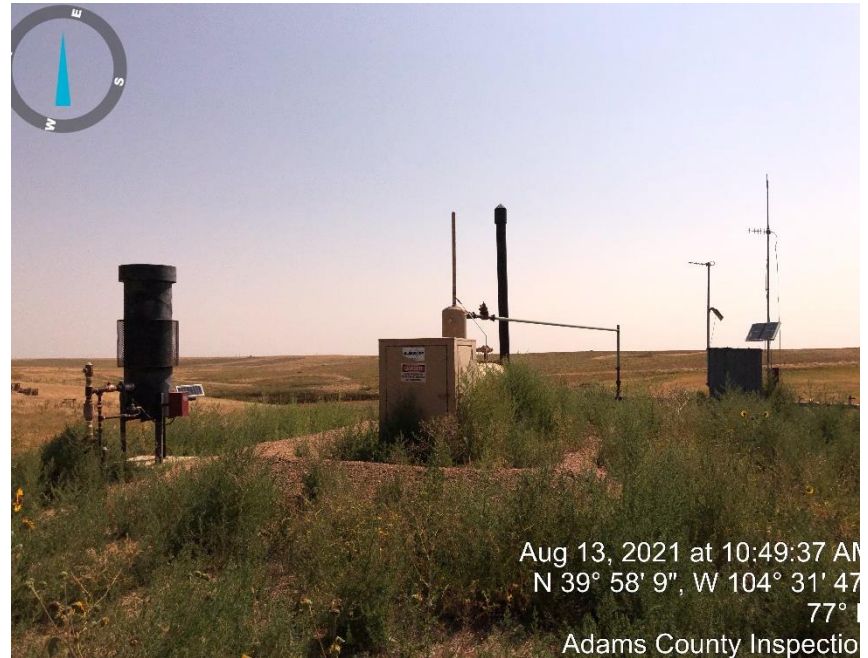
Photo #2 ECD, Separator & Meter.
