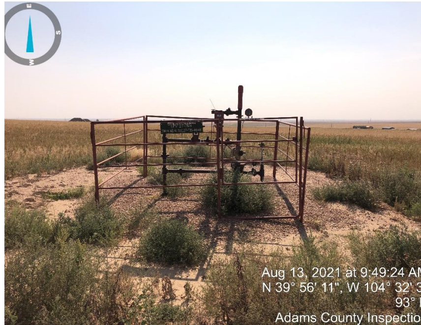
Photo#3 Well Head.
