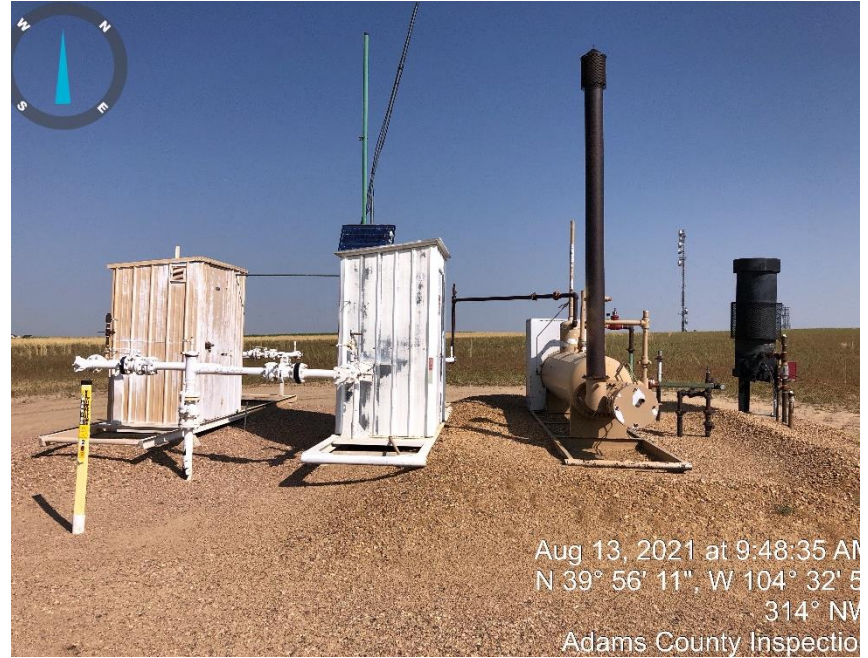
Photo #2 ECD, Separator & Meters.
