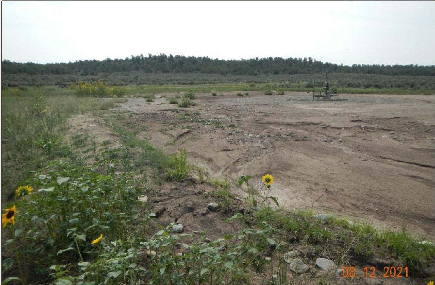
Photo 1. View of the southern portion of the working area from the western edge facing center. Stormwater flows over the well pad largely appear contained by a silt trap along the western edge. Monitoring and maintenance will be needed to maintain site stabilization due to site layout.
