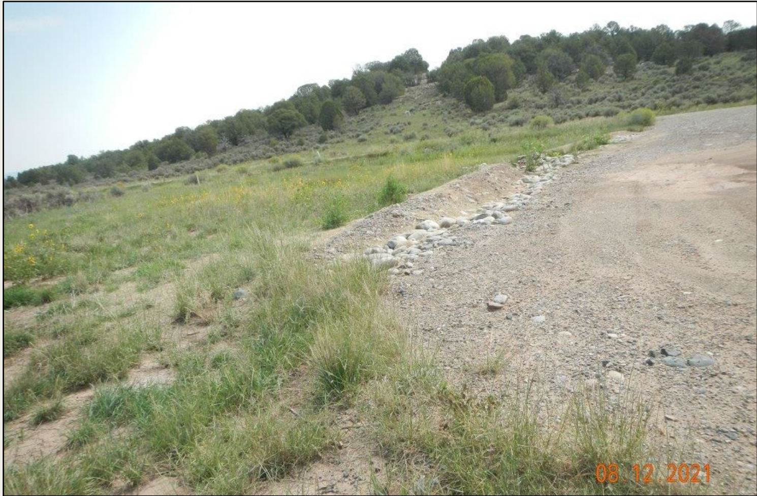
Photo 2. View of the northern project area from the northwestern corner facing eastward. Reinforced berms and silt trap are installed.
