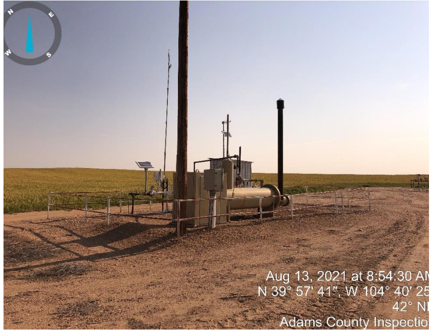
Photo #2 Separator & Meter.
