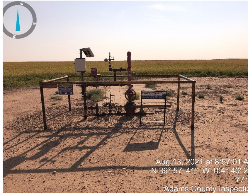
Photo #3 Well Head.
