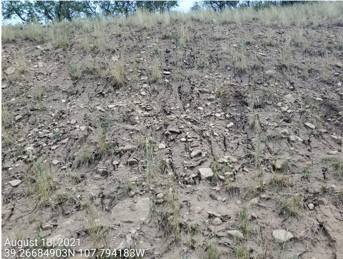
Photo 2: Photo taken from the west end of the Location. Photo shows areas where uniform establishment is not occurring and inter-seeding is needed. Photo also shows BMPs to stabilize the slopes are missing or insufficient.
