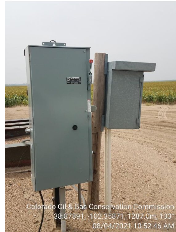
2. Elec panels, Cathodic rectifier
