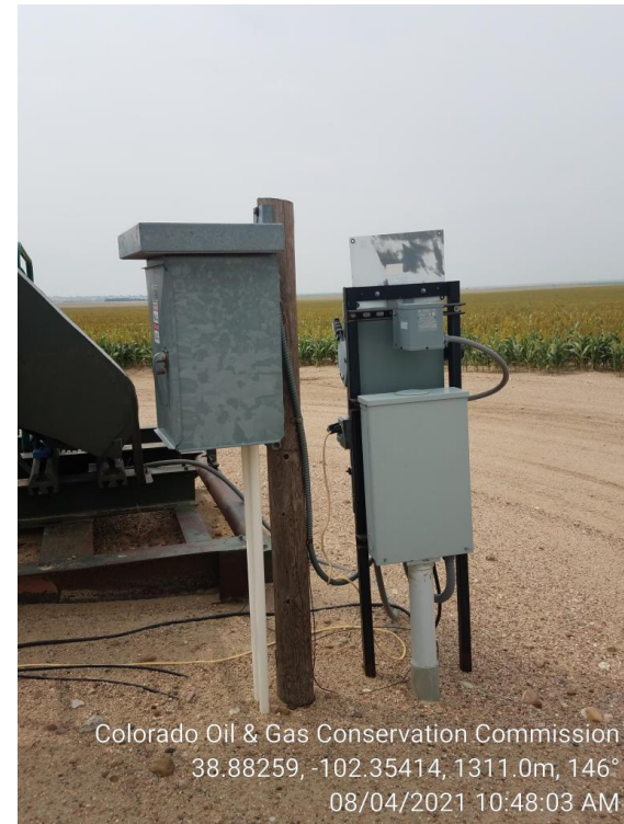
2. Elec panels, Cathodic rectifier, Prime mover
