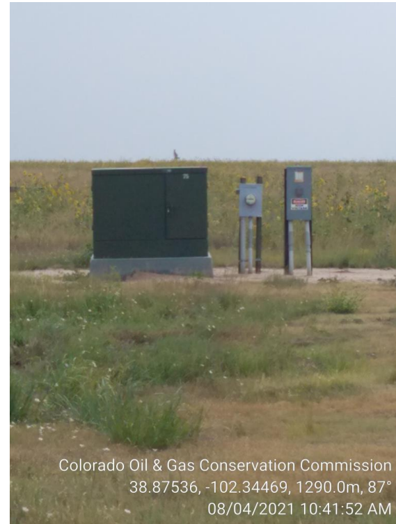
2. Elec Meter, Panel, Transformer
