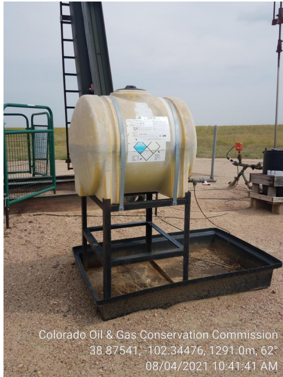
3. Chemical Tank W/BMP
