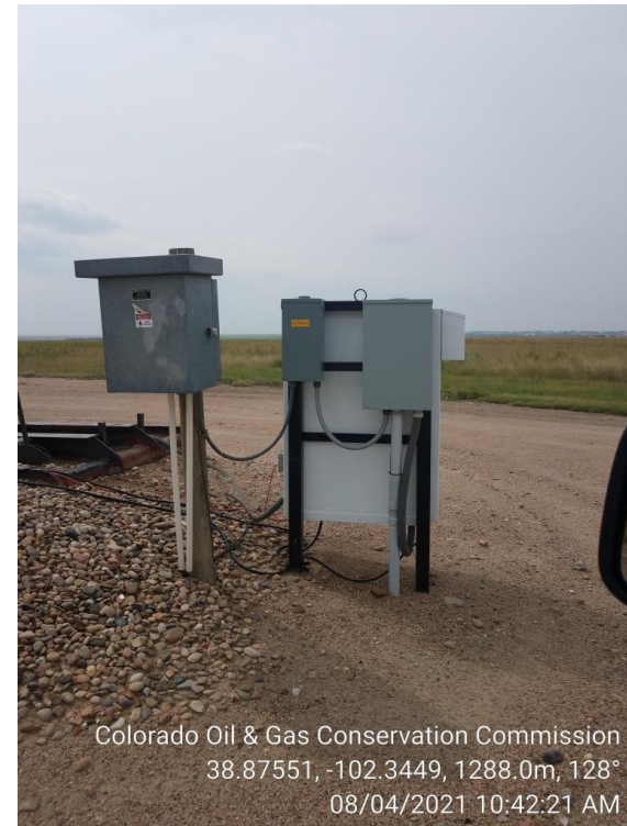
2. Elec panels, Cathodic rectifier
