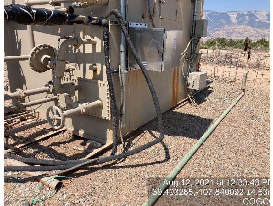
Lack of separator bath signage
