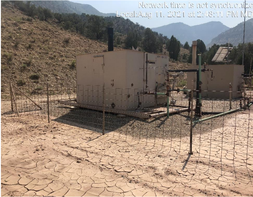
Photo #4768 Separator missing required information.
