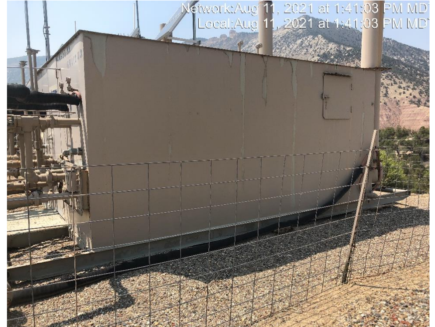
Photo #4759 Separators missing required information.
