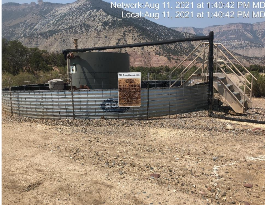
Photo #4758 Battery sign weathered and not legible.
