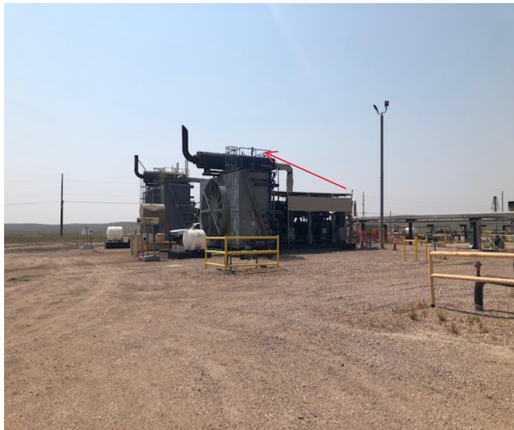
Source Area Red arrow indicates failure point
