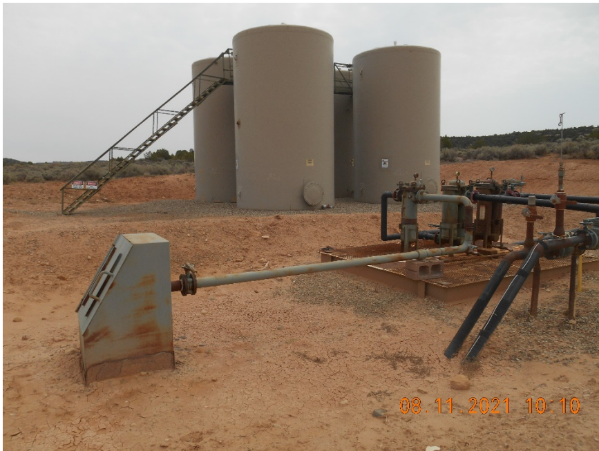
Loading station and Filter pod
