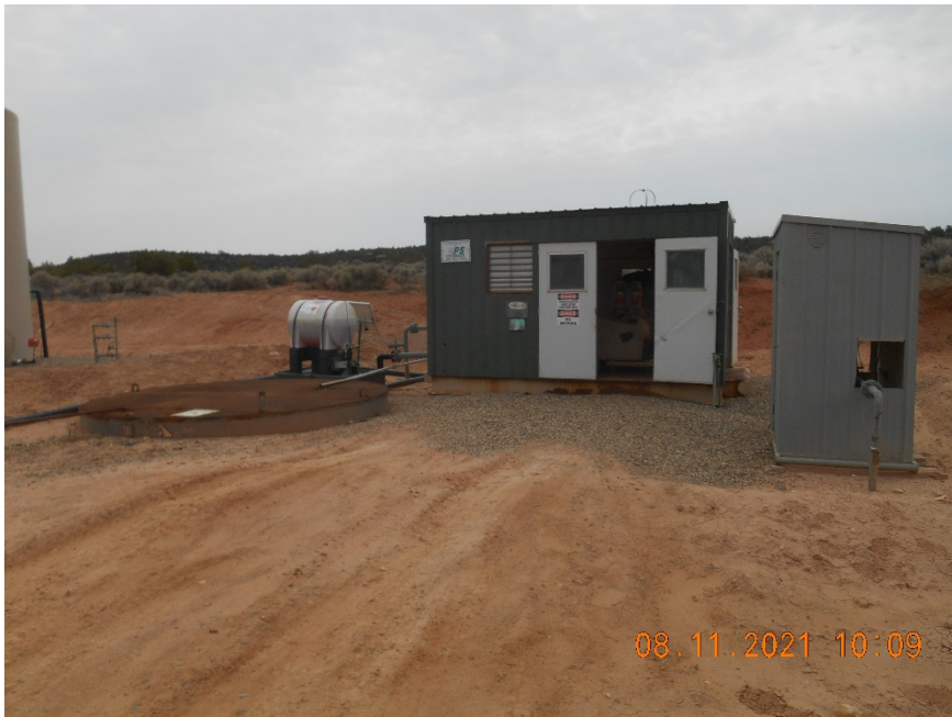
Pump housing. Meter shed.
