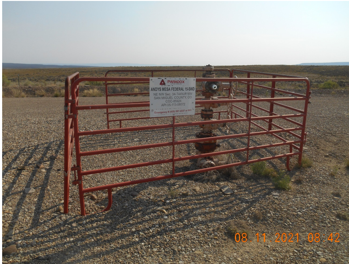
Injection Wellhead – Temporarily Abandoned
