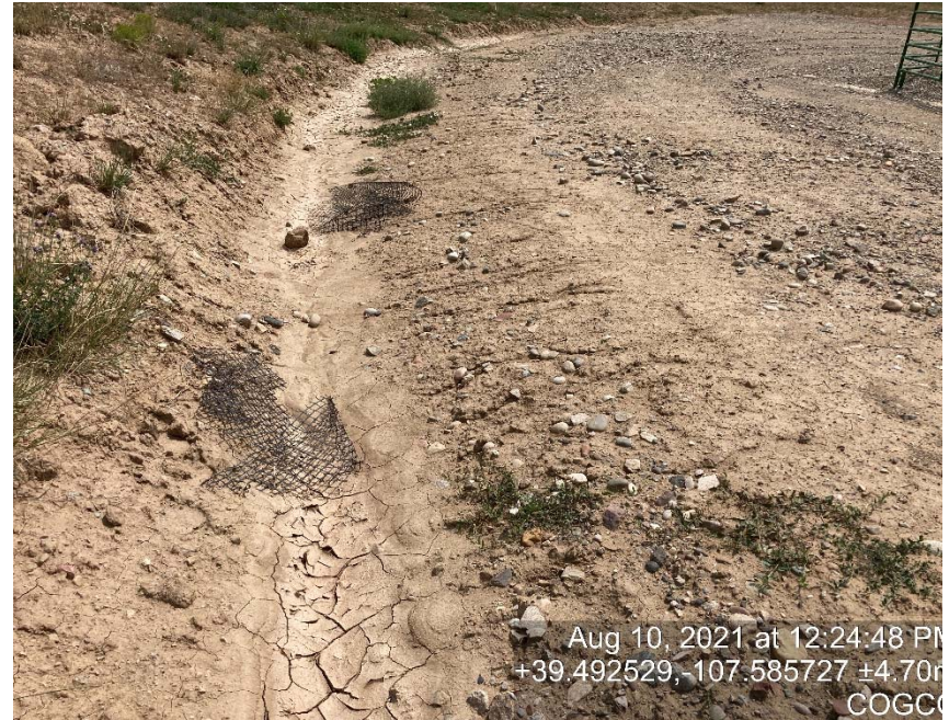
Follow up inspection photo of ditch around location (debris)
