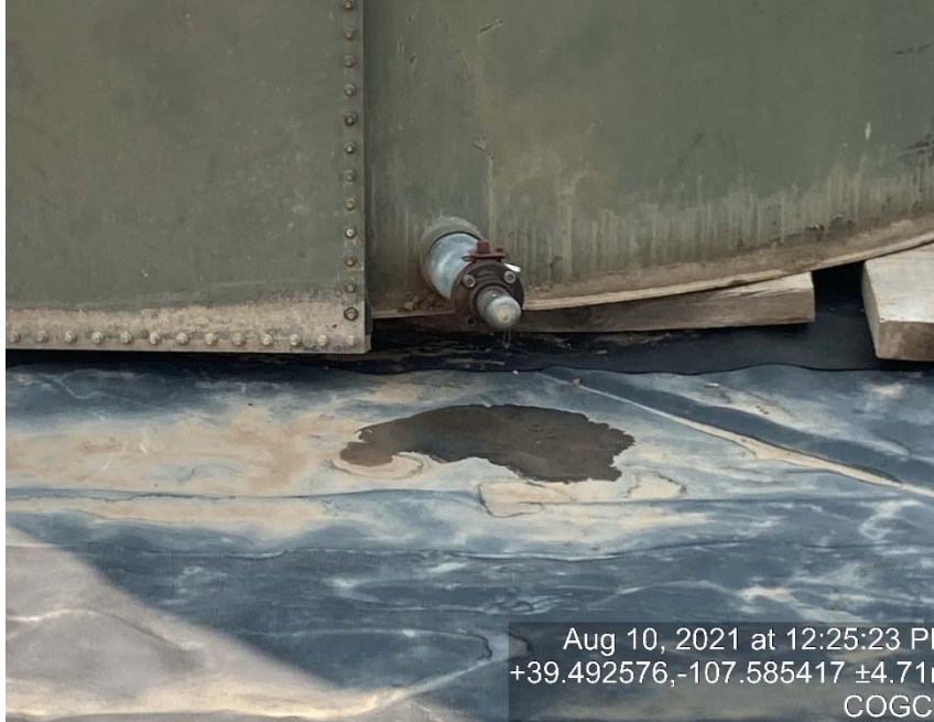
Staining under tank valve
