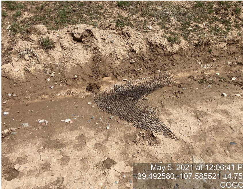
Previous inspection photo of ditch around location (debris)
