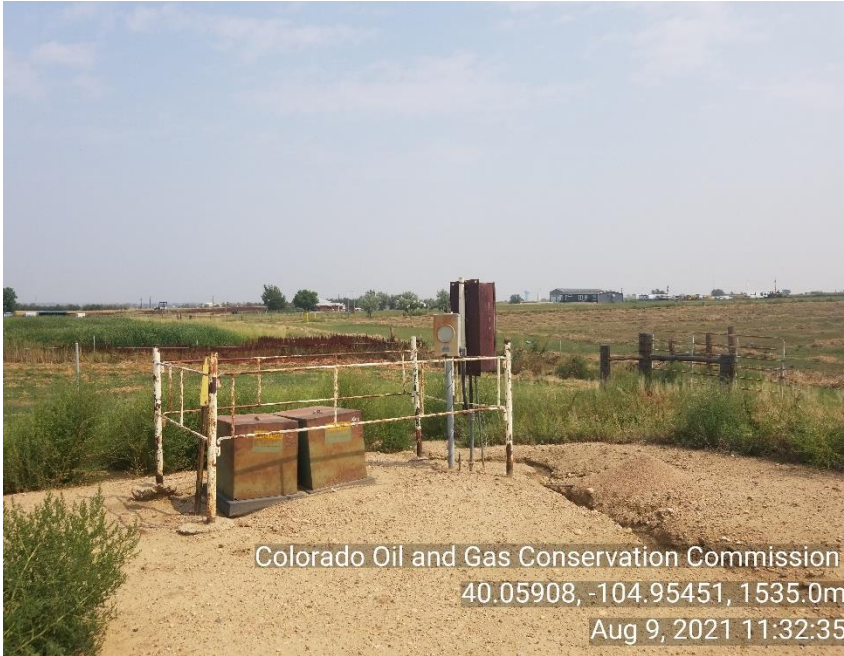
Photo 3 Meter has been pulled from electric panel.
