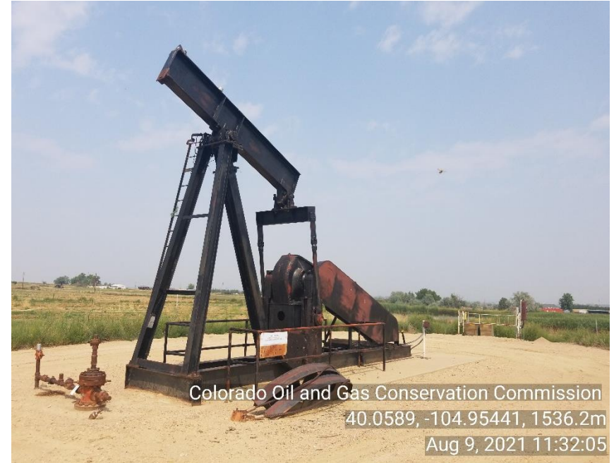
Photo 2 well is TA Unused equipment PU and electric panel.
