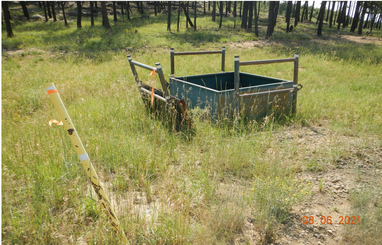
Photo 1. The valve box lid is open at the road intersection adjacent to the location. This needs to be closed to prevent entry.
