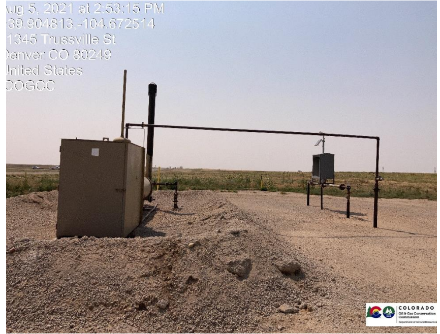
Pic 2 separator, gas meter run.
