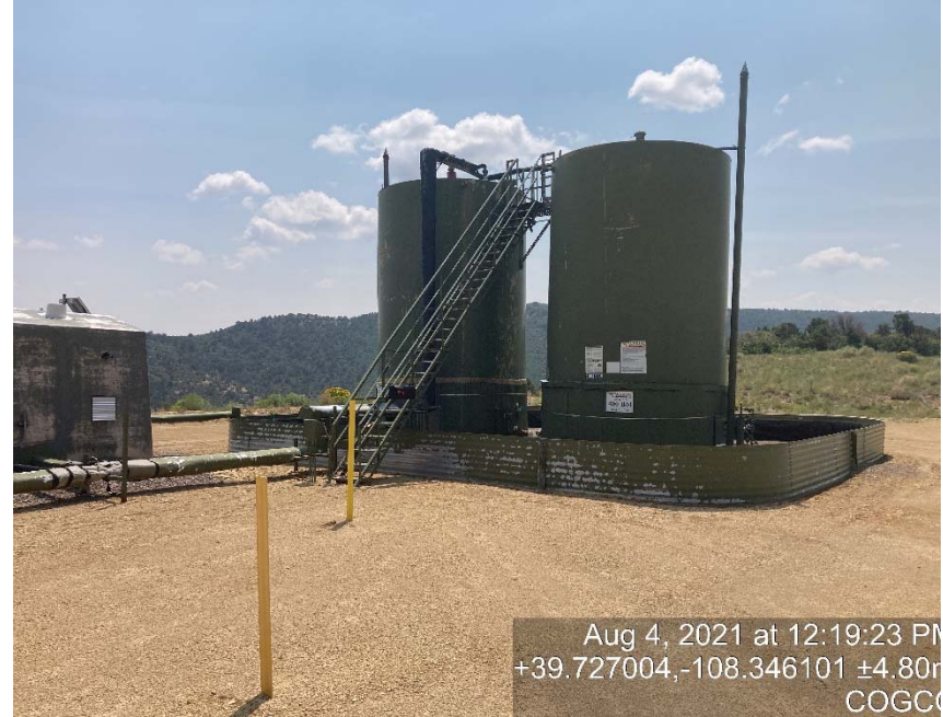
location/lack of battery signage
