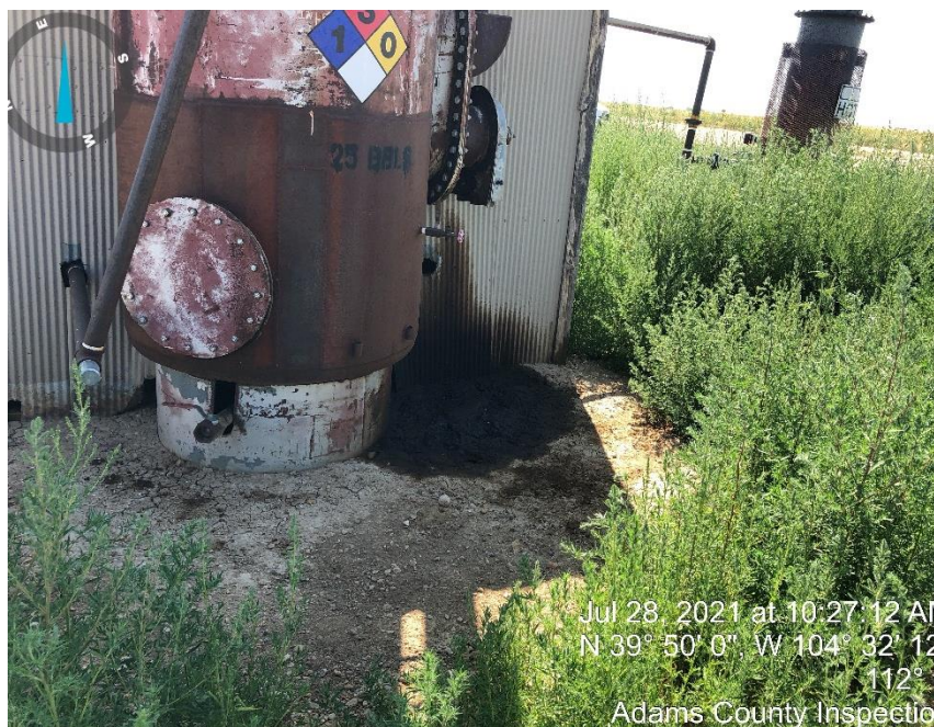
Photo #5 stained soil in west side of separator.
