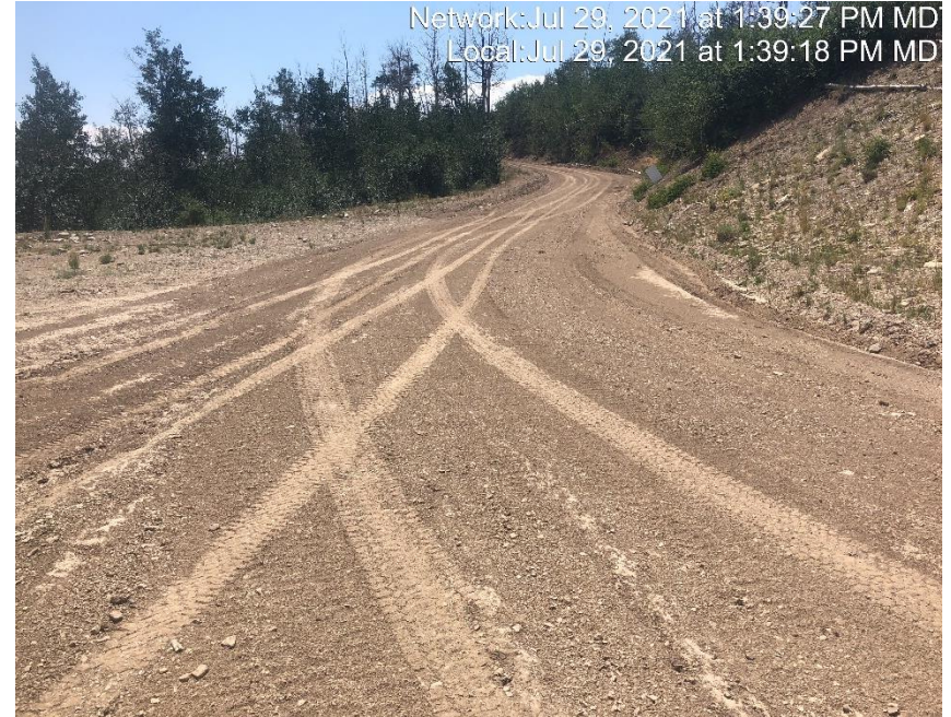
Photo #4616 No form of tracking BMP located at entrance to location.
