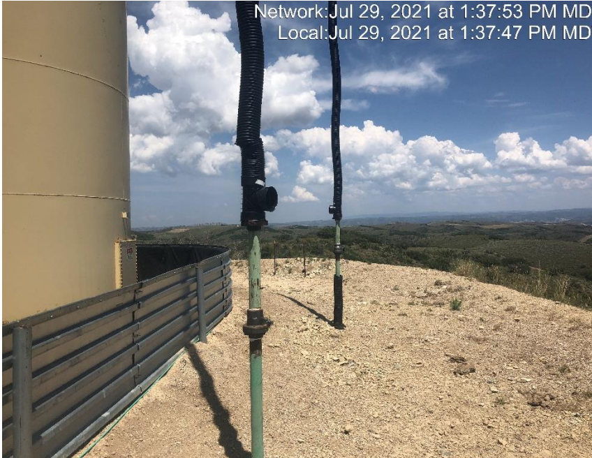
Photo #4613 Multiple flow line heating insulation open ended and not capped.
