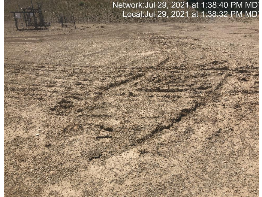
Photo #4614 Location lacks stabilization.
