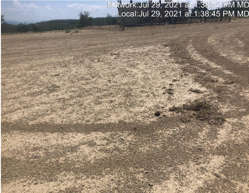
Photo #4615 Location lacks stabilization.
