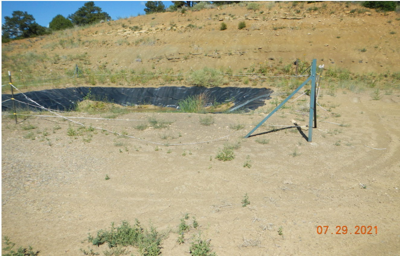
Photo 2. The fence around the pit is not maintained. This issue has been previously observed and needs adequately fenced and maintained.
