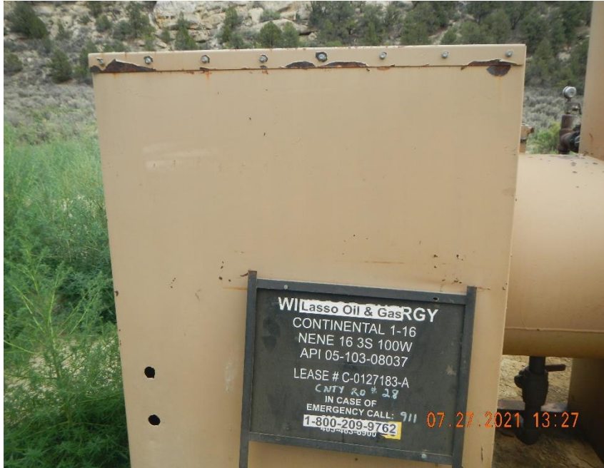
Well sign is leaned up against separator.
