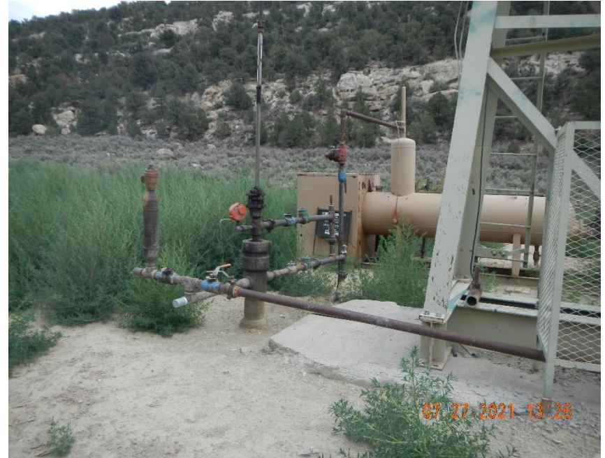
Weeds around well and separator.
