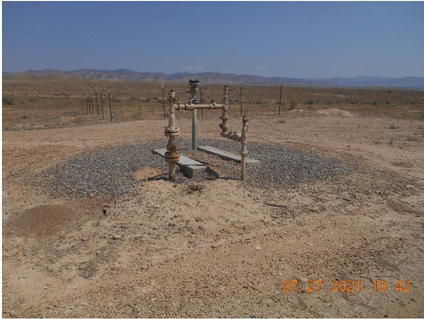
Separator risers locked out/tagged out
